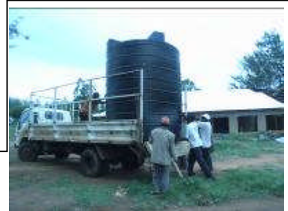
Delivery of 10000L tank. To be placed on a stand to be the feeder tank to the homes. The workers could hardly believe their eyes when they saw it
