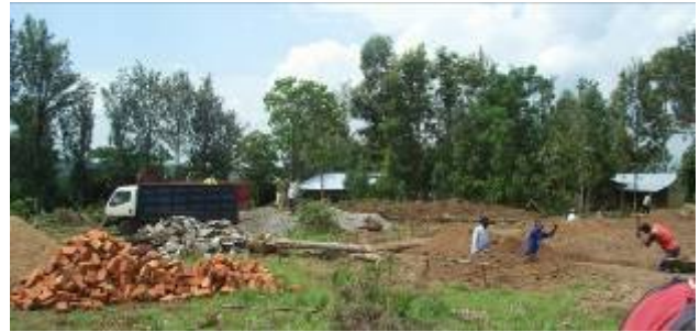
Men digging foundations to the right. Materials being delivered to the left. In the background to the left you can see the brick shelter and the Building to the right is the small cottage already on the site that we will Renovate to be office space and living quarters.
