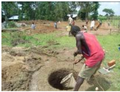
Water being drawn from the well. Another worker is down in the hole.
