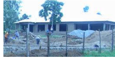
The roof is almost complete. The foundation for the second house is in the foreground.
